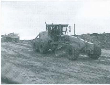
Left: Regular grading on internal haul roads can help reduce tyre wear, but increase the proportion of small particles on the surface, and consequently the potential for dust release.
